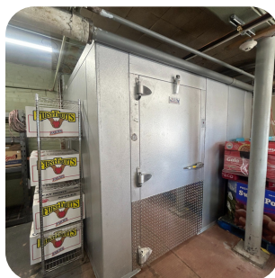
New walk-in freezer & fridge make it possible to store large quantities of fresh produce.
